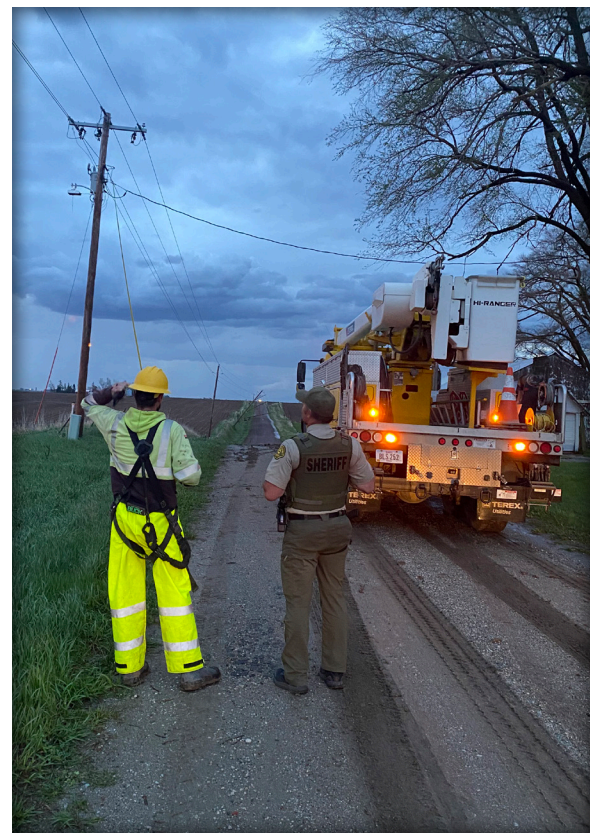
Crews from Midland Power Cooperative joined NVREC crews to restore service after the April 26 storm.
